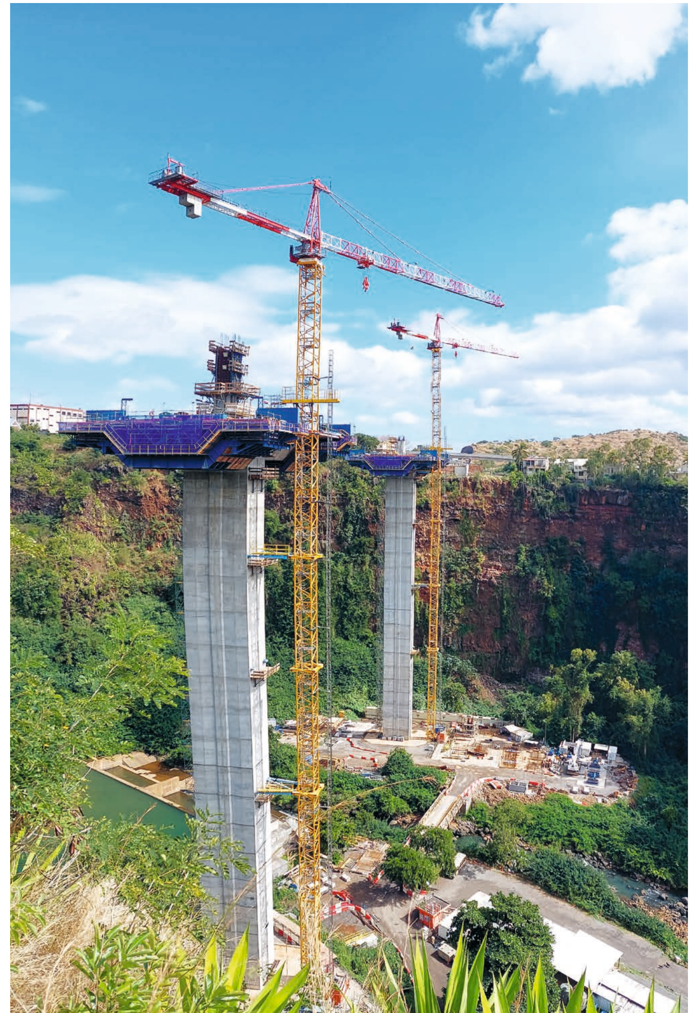
When completed, the bridge will link two of the country's most important motorways.
