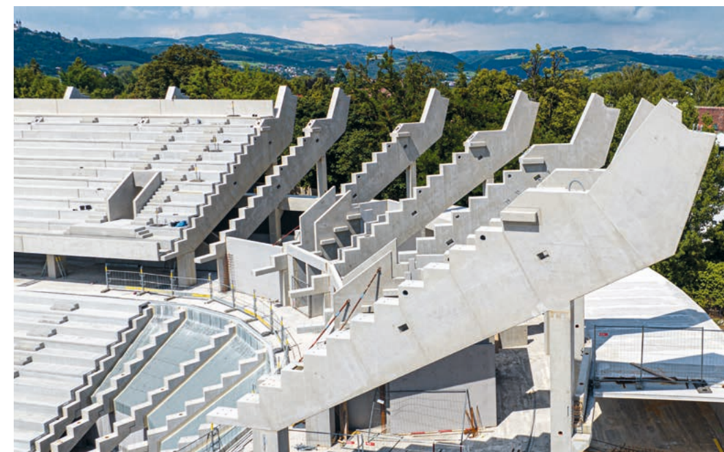
1, 2, 3 Doka played a leading role in the construction of the new Linz stadium, supplying the grandstand pillars.
