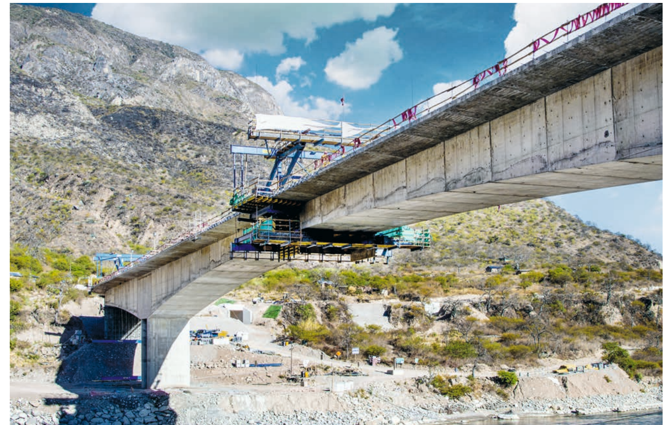
1, 2 Closing segment of the bridge over the Rio Pampas, forming a stable structure with two cantilevers.
