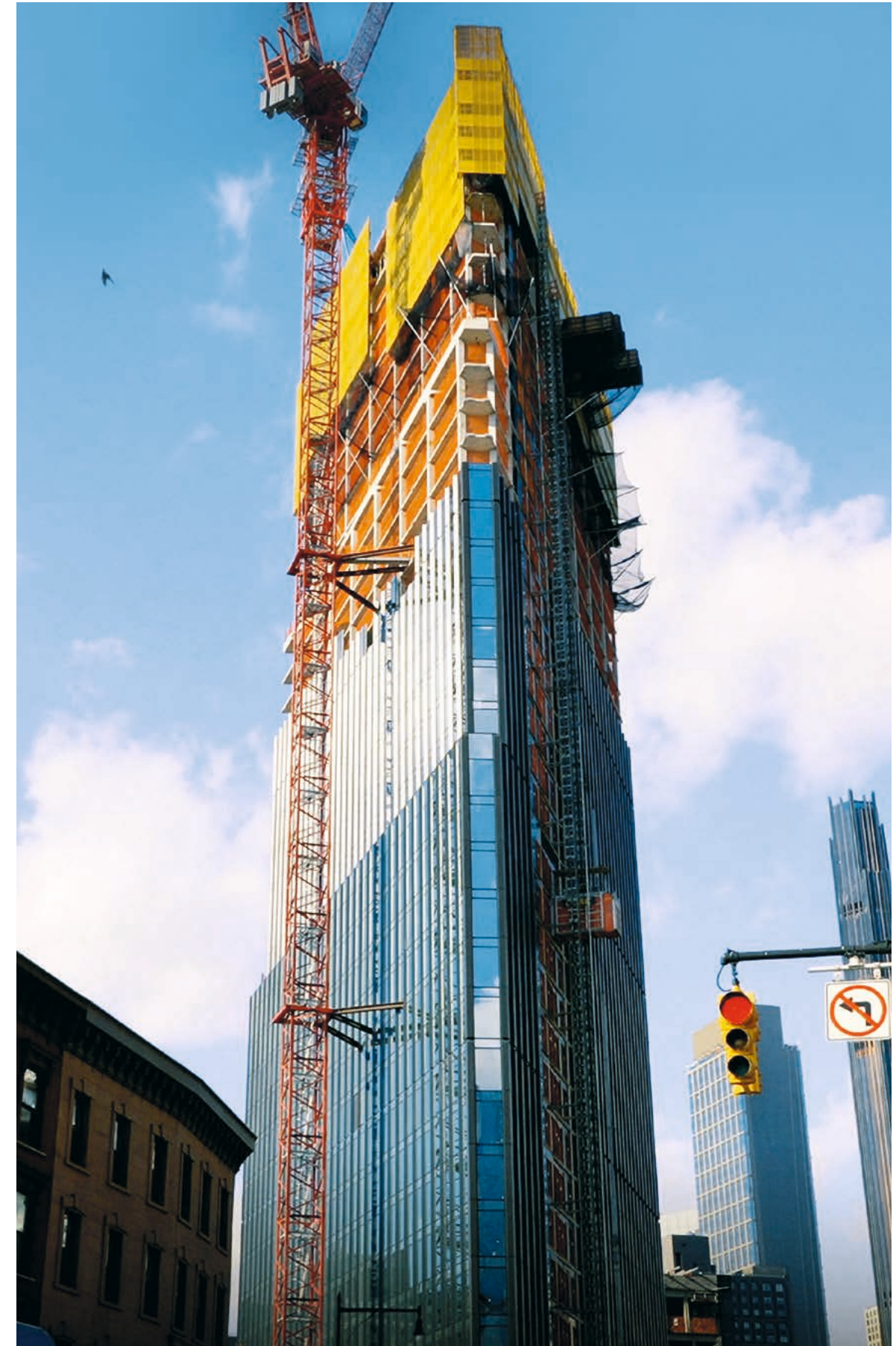
Doka's Xbright protections screen solution ensures full safety around the entire perimeter of structure to ensure worker safety.
