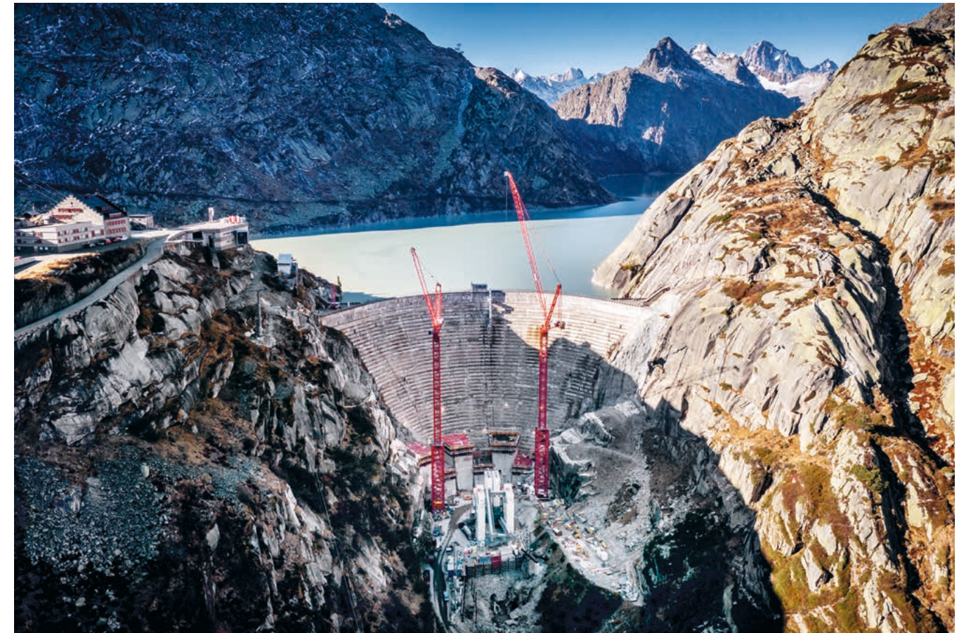
1 The Spitalamm Dam construction showcases how Doka is harnessing digital services and legacy knowledge to help customers improve efficiency and safety.
