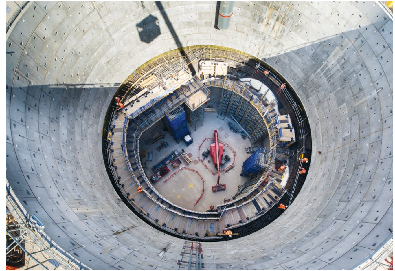
1, 2 Due to the shaft's height and its huge 25.1 m radius, the concrete needed to be cast in stages.
