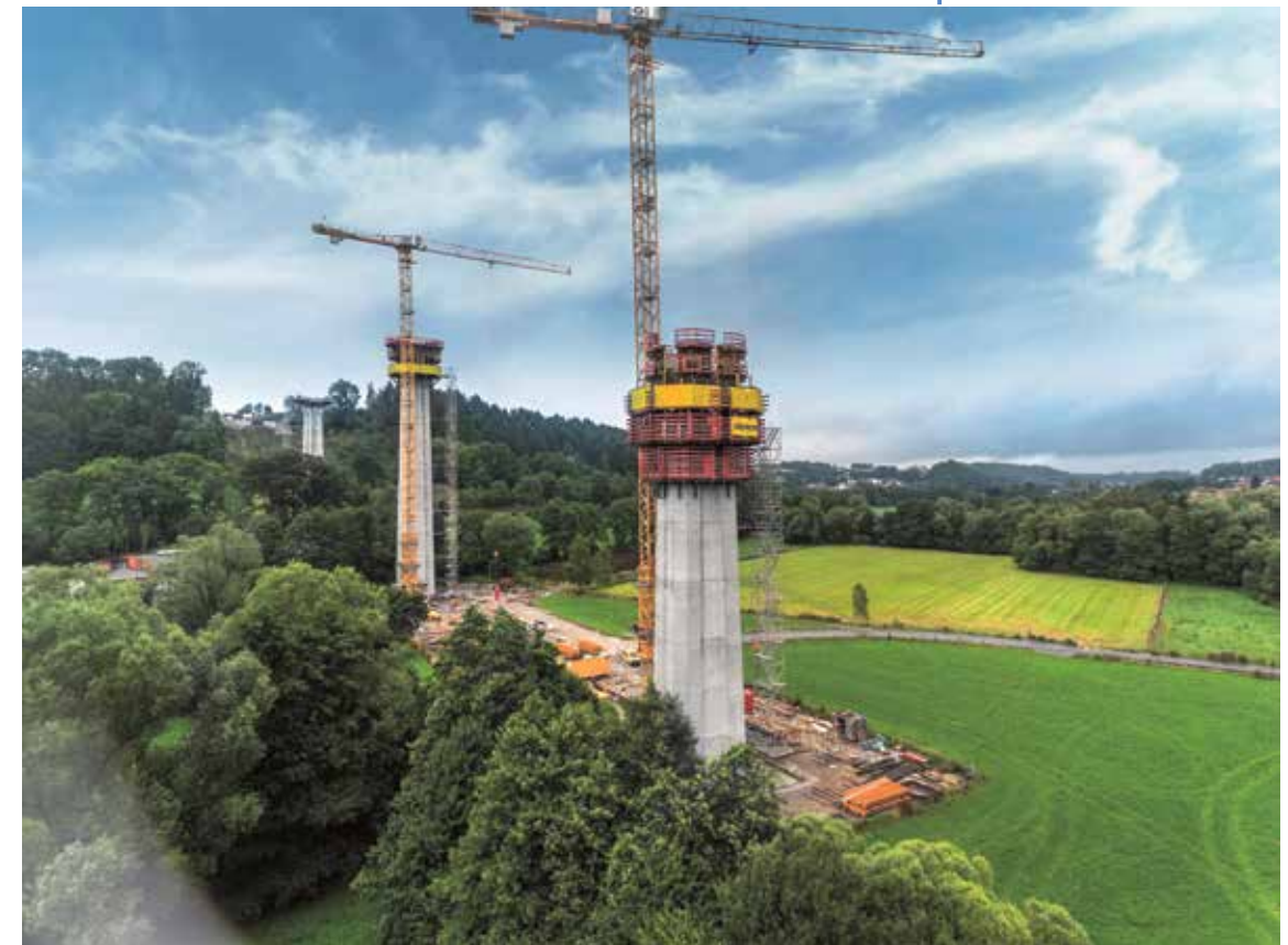
2 The viaduct is supported by six piers, some of which reach a height of up to 66 metres.
