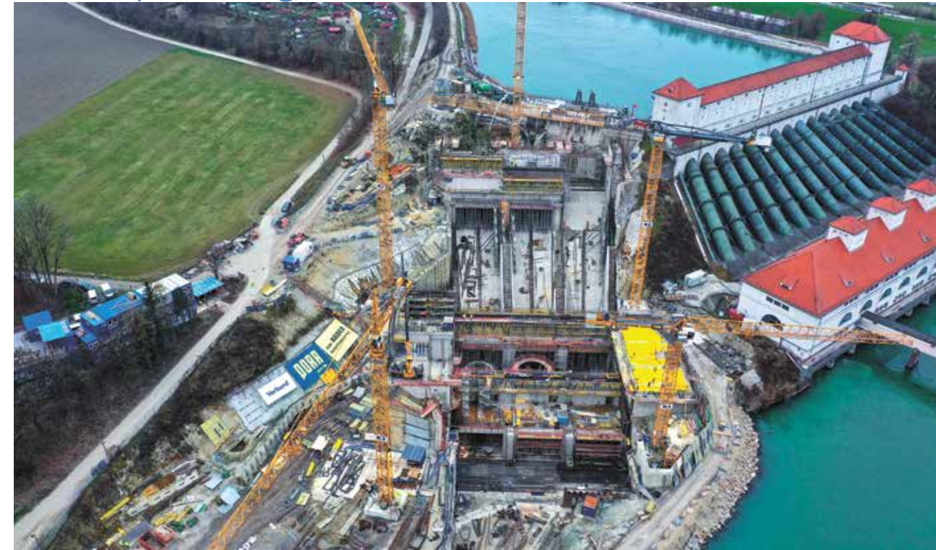
1 The new, highly efficient Töging power plant is being built beside the existing historic power plant. ©Kasjan Choroba
