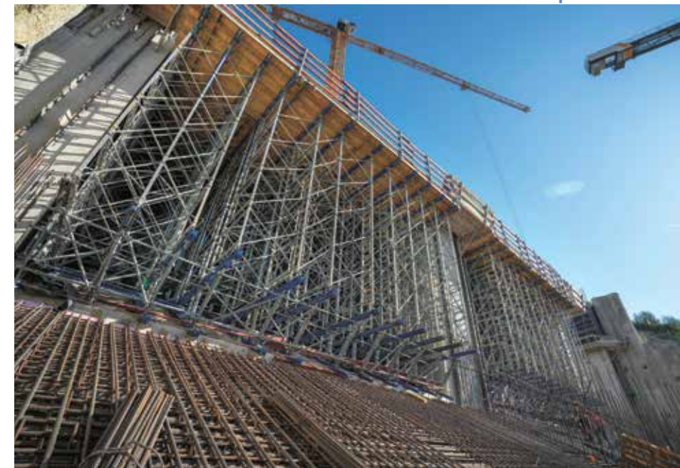
2 Around 1,400 frames of the Load-bearing tower Staxo 100 were used for the inlet structure.
