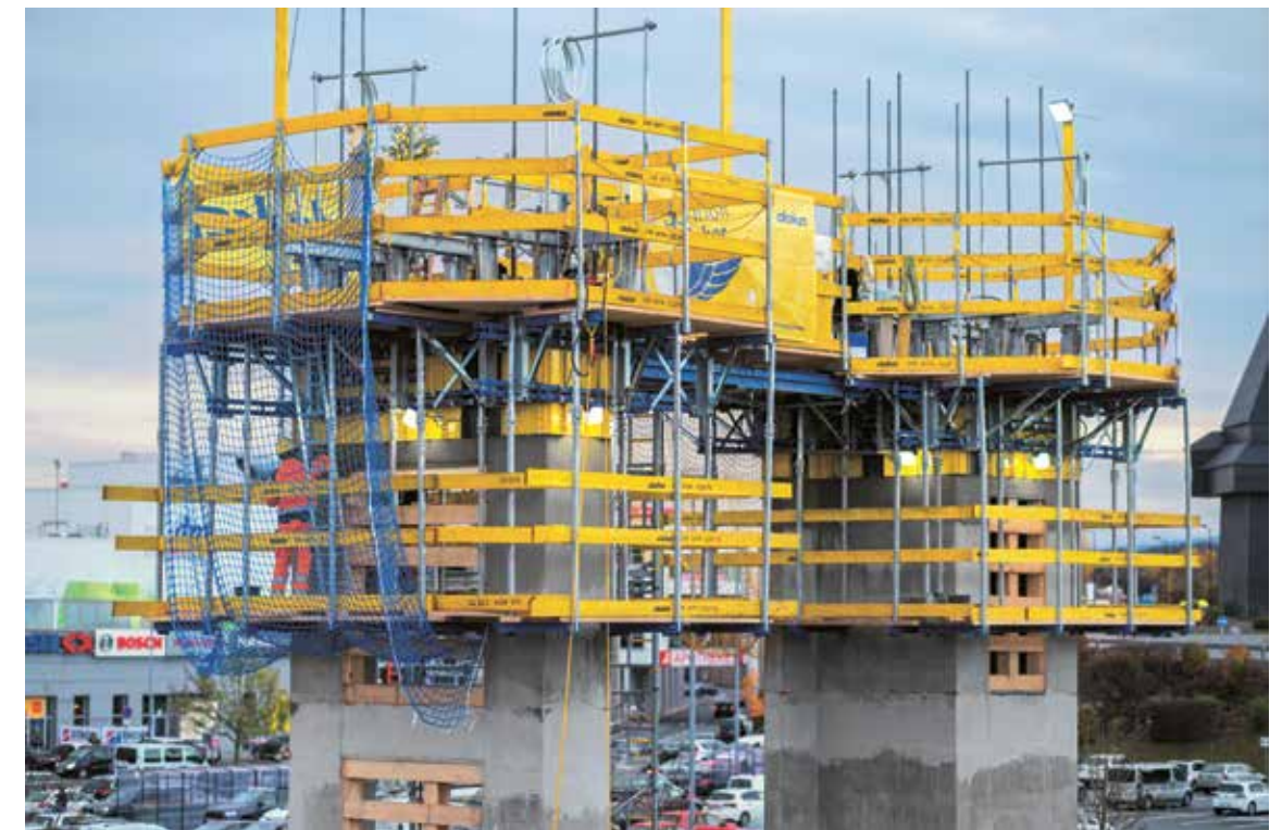
2 The slipforming method allows concreting 24/7, which means that high construction projects can be erected quickly and economically.
