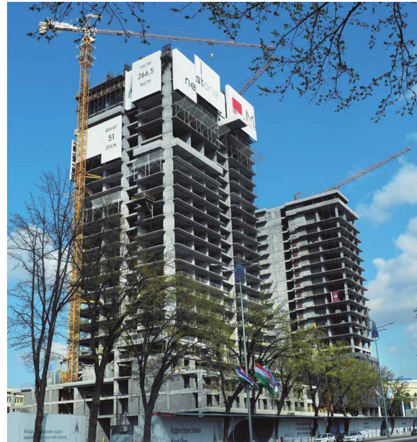
1 With 56 storeys, the Nest One multi-purpose building will reach a height of 266.5 metres.
