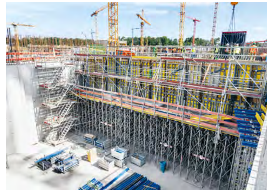
Quality was also crucial when it came to ensuring safety: Three quarters of Doka's entire European stock of Staxo 100 scaffold decking was used here to ensure safe access.
