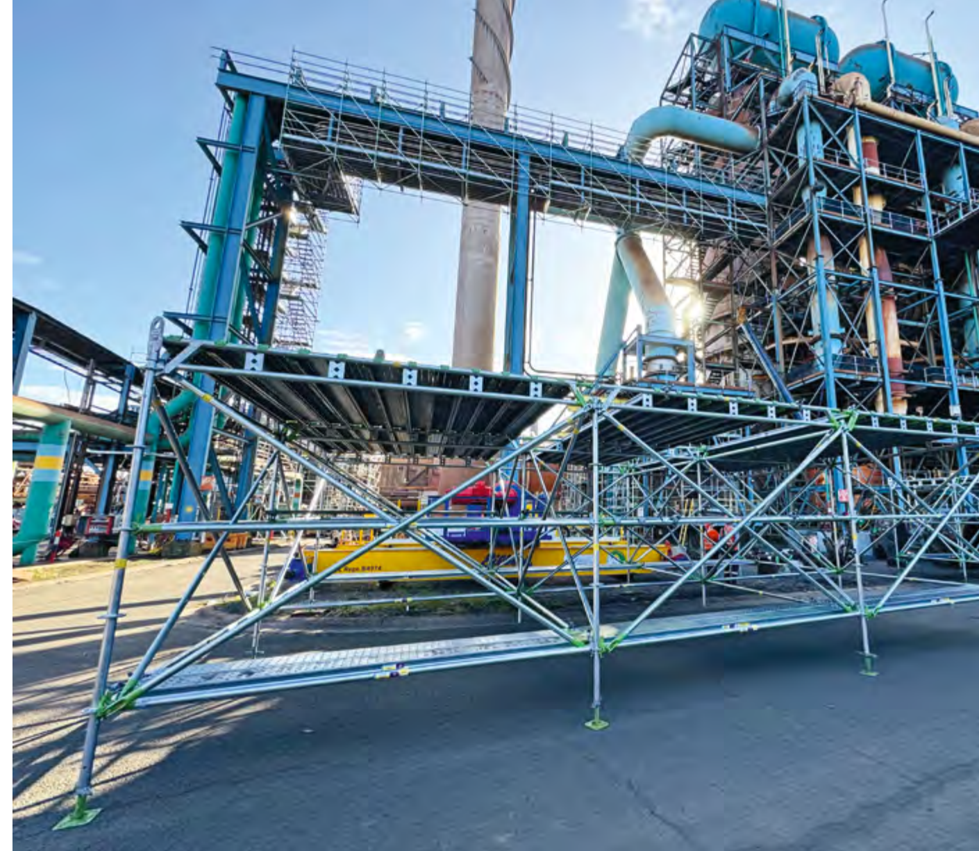
BlueScope operates the Port Kembla steel mill in New South Wales, Australia. The Industrial Scaffold Ringlock is currently being utilized for the works on the environmental upgrade.
