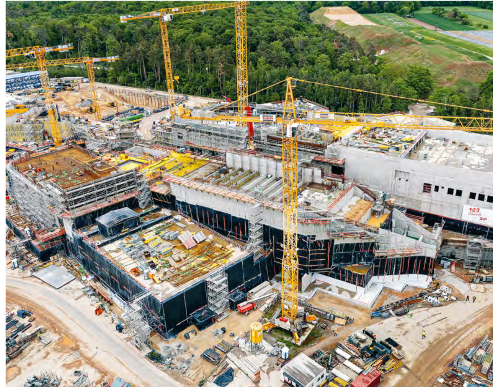
The FAIR particle accelerator centre is being built in Darmstadt. Züblin and Doka are also involved in this gigantic construction site.
