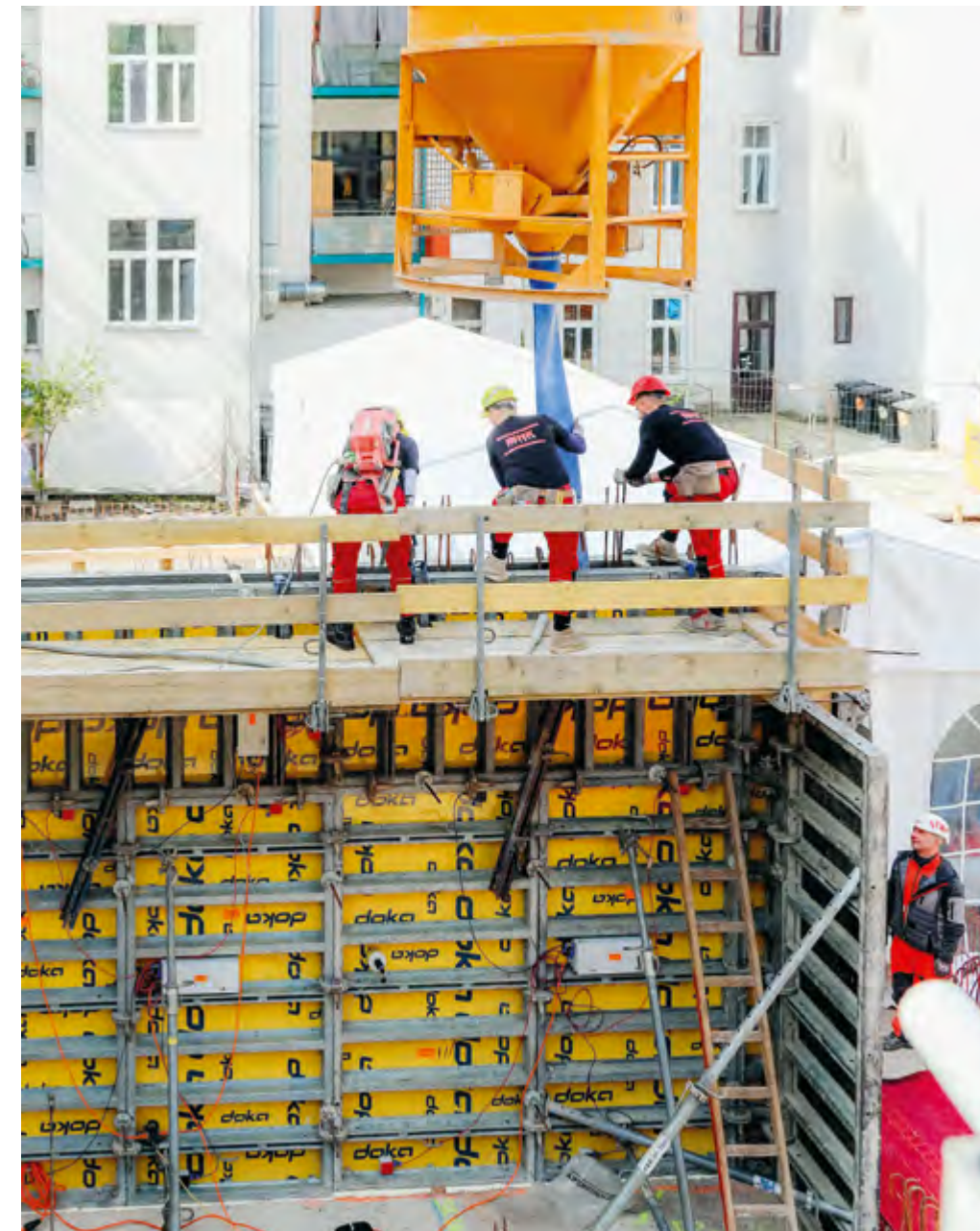
Flagship project in Vienna: first-time use of CO 2 -reduced concrete (RCC) in a residential project by STRABAG Real Estate. The Doka prototype is being used to build the walls in the basement and on the ground floor.
