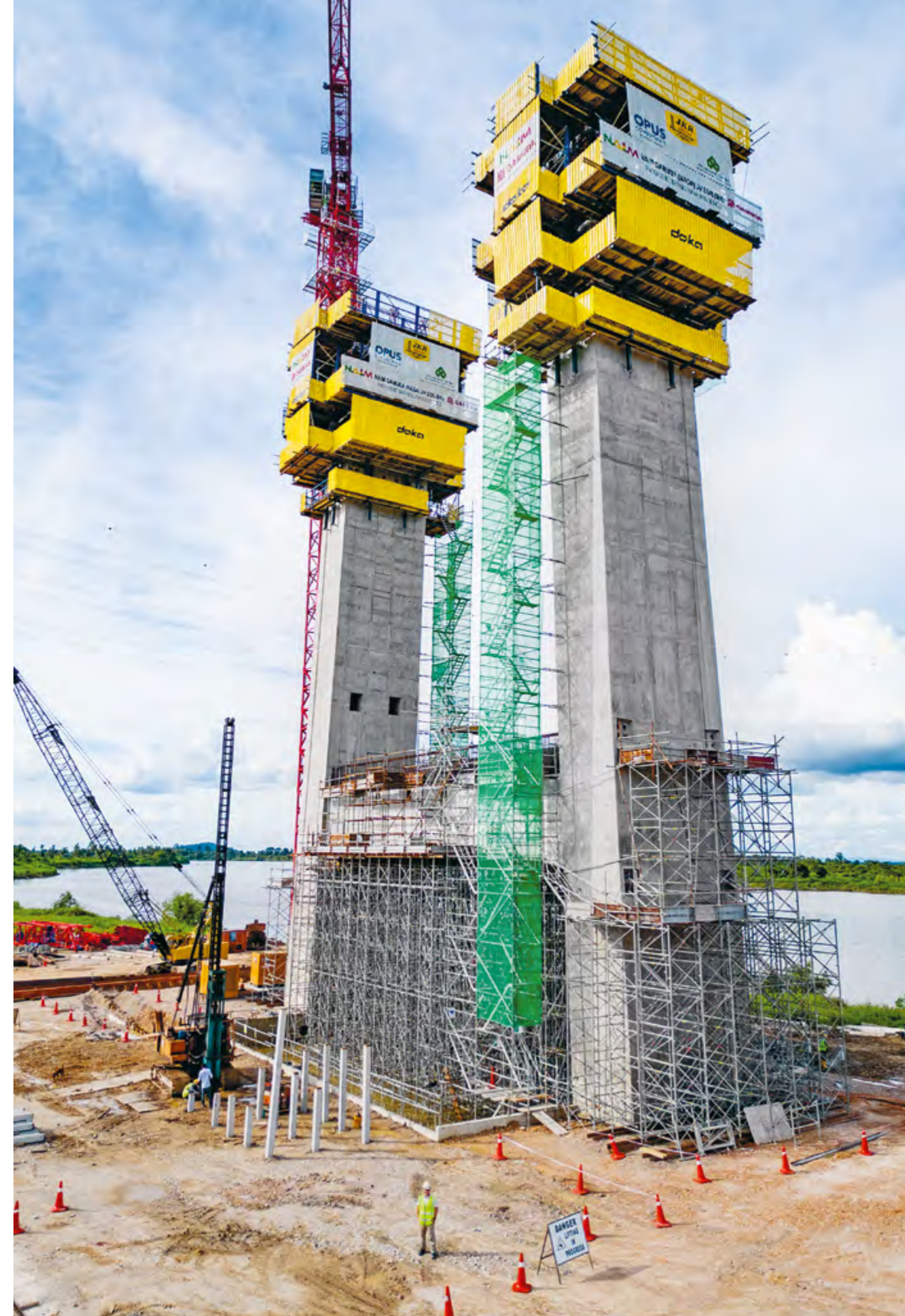
Doka's Ringlock and Automatic Climbing Formwork SKE 100 plus in action as progress continues on the western pylons.
